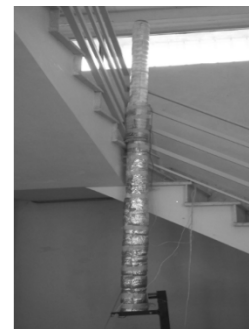
Fig. 9. A picture of the vertical insulated pipe.
